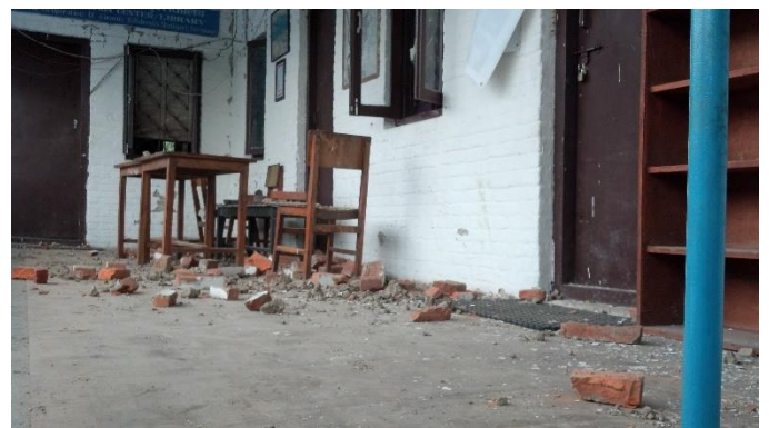
Tri Ratna Cooperative School in Bungmati, School has been immensely damaged by the Earthquake
